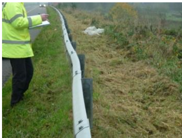
Figure 4.10 - Low priority defect: no posts broken or detached, deflection < 150mm
