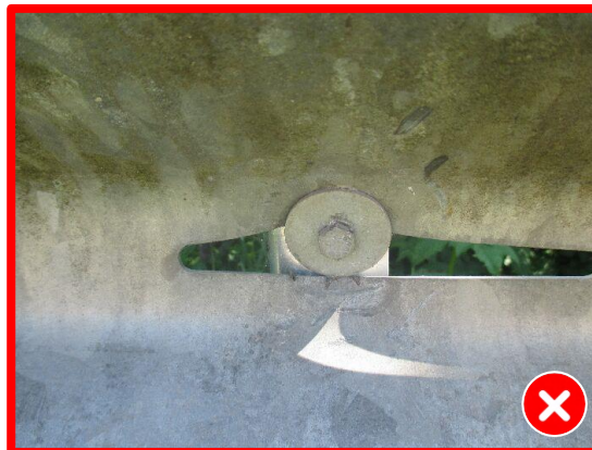
Figure 4.16 - Unacceptable deformation at beam to post connection slot
