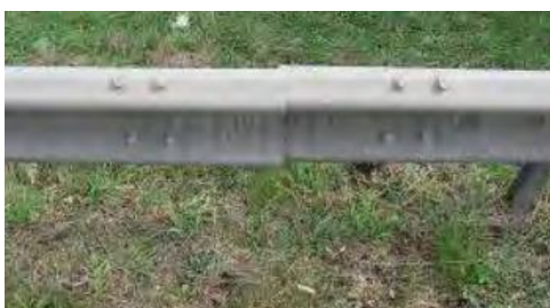
Figure 4.5 - High priority defect: loose beams, poses risk of VRS failure and sparring
