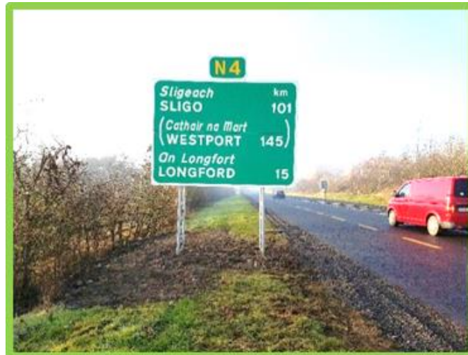
Figure 4.3 - Sign installed on passive posts to enable complete removal of defective VRS
