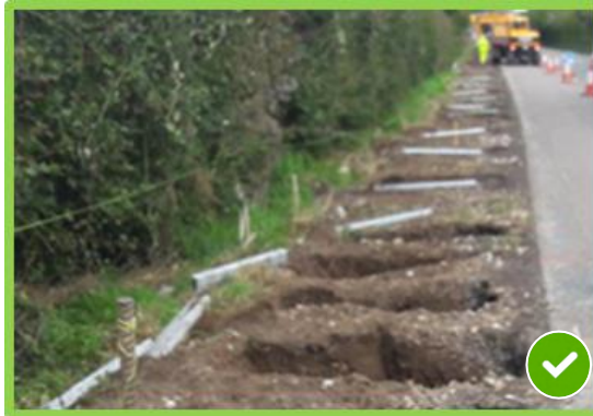
Figure 3.13 - Example of hold point, where dug foundations must be inspected prior to pouring concrete
