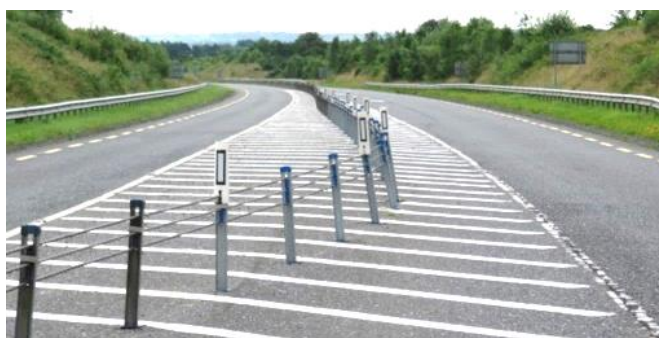
Figure 4.7 - Medium priority defect: wire rope posts leaning due to tension
