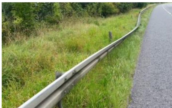
Figure 4.6 - High priority defect: beams detached from posts
