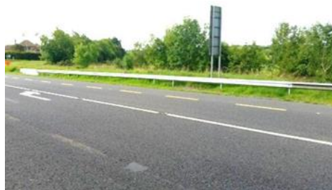
Figure 2.9 - Example of system progression to connect new replacement terminal and W2 transition to existing W5 barrier
