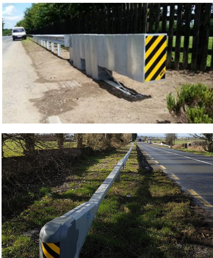
Figure 3.18 - Examples of prEN1317-7 terminal and transition installed as part of a VRS repair
