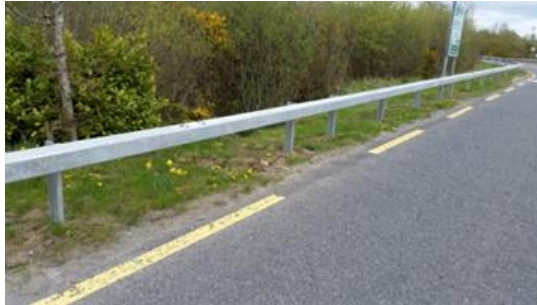
Figure 5.7 - Unacceptable post centres due to incorrect setting out
