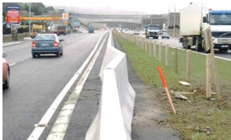
Figure 3.9 - Example of 'High Priority' Damage to precast concrete VRS (significant displacement > 60mm)
