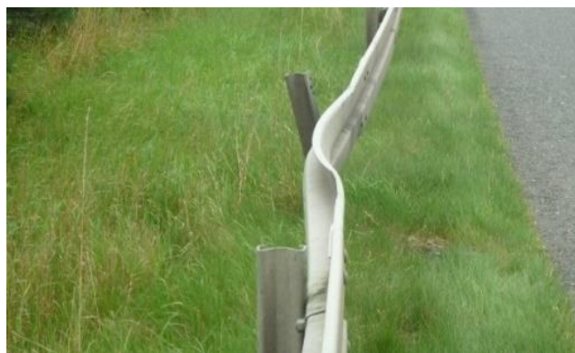
Figure 4.8 - Medium priority defect: single post damaged, beam slightly bent, deflection < 300mm
