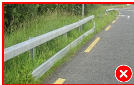
Figure 3.3 - Example of VRS damaged beyond function, but has not been made safe
