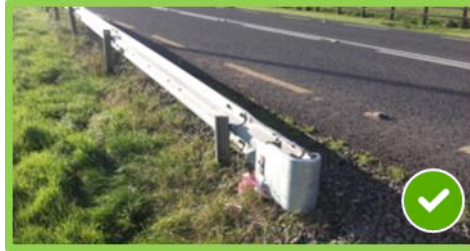
Figure 3.5 - Example of damaged VRS at low risk location treated with temporary ramped beam and end plate to reduce risk of spearing
