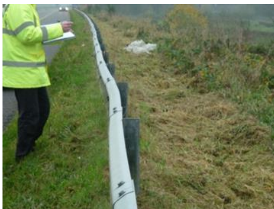
Figure 3.11 - Example of 'Low Priority' Damage (no posts broken or detached, deflection < 150mm)
