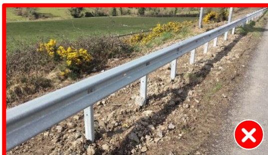
Figure 5.16 - Poorly reinstated following VRS repair works – uneven, large stones, not seeded
