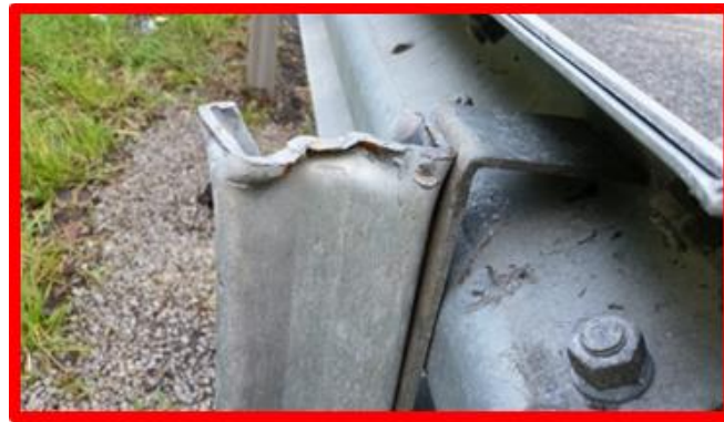
Figure 3.27 - Unacceptable damage to post from driving rig
