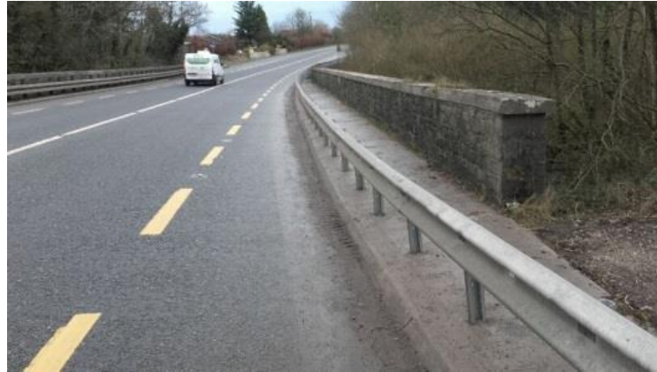
Figure 4.15 - Inadequate setback following pavement overlay and verge works
