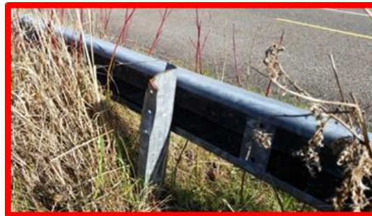
Figure 4.22 - Post structurally damaged due to verge maintenance activities
