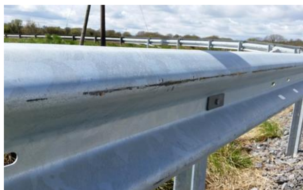
Figure 4.9 - Low priority defect: zinc coating damaged
