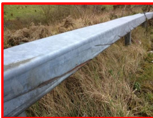
Figure 4.24 - Deep scratches with evidence of corrosion, beam should be replaced
