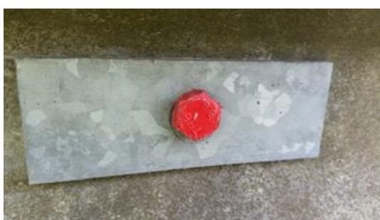
Figure 5.6 - Grade 8.8 bolt used when grade 4.6 was specified – installation not covered by manufacturer's warranty
