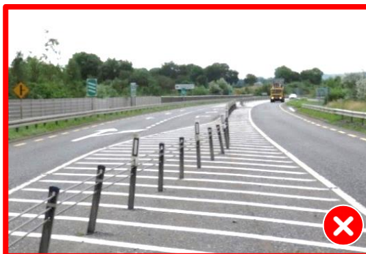
Figure 4.23 - Series of posts out vertical tolerance due to incorrect radius used on alignment
