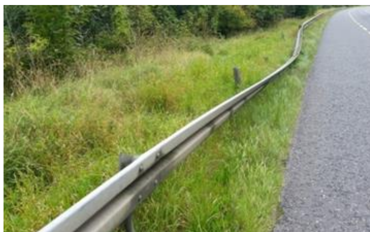
Figure 3.8 - Example of 'High Priority' Damage (beams detached from posts)
