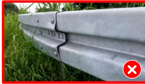
Figure 2.7 - Incorrect radius beam used in a repair
