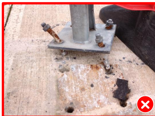
Figure 5.11 - Inappropriate fixing resulted in surface mounted post baseplate pulling away during impact
