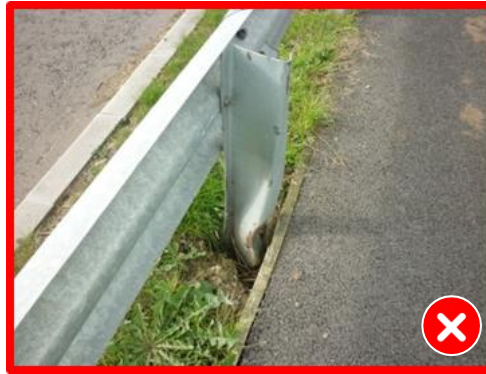
Figure 2.5 - Structurally damaged post should be replaced
