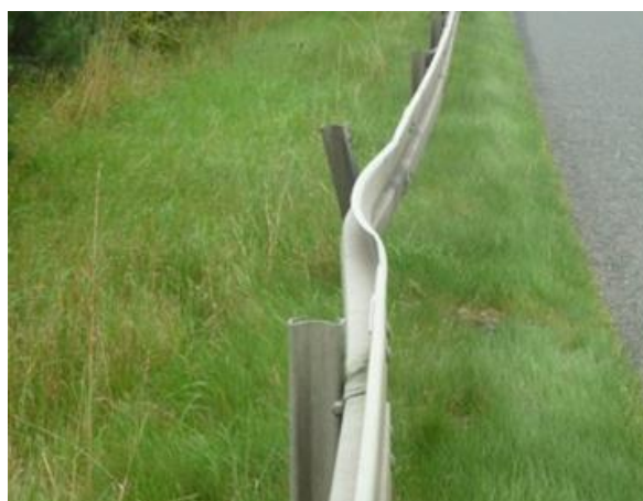
Figure 3.10 - Example of 'Medium Priority' Damage (single post damaged, beam slightly bent, deflection < 300mm)
