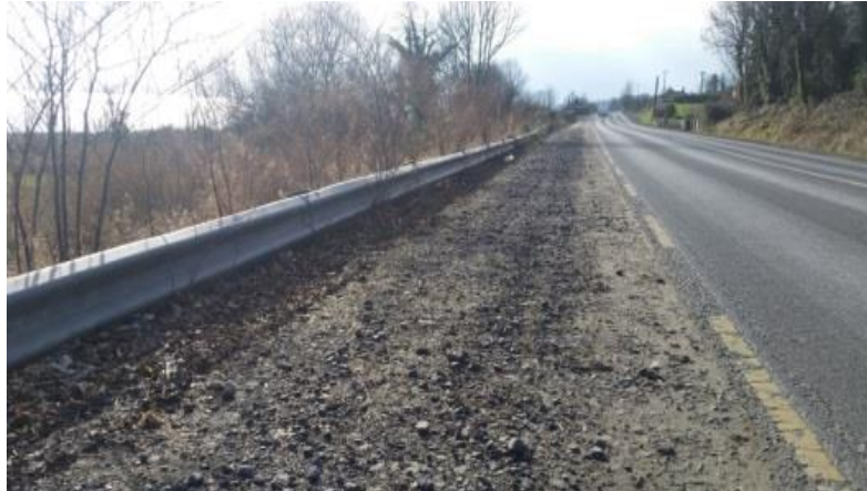
Figure 4.13 - VRS too low and out of spec due to pavement overlay
