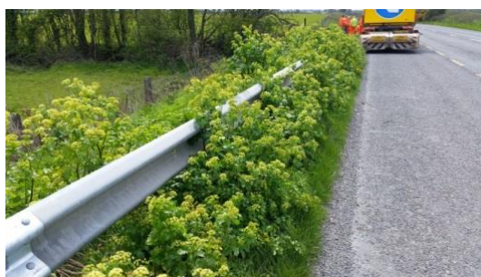
Figure 4.25 - Barrier cannot be fully inspected due to vegetation
