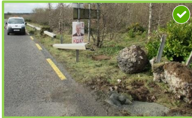
Figure 3.28 - Damaged posts with concrete footings removed, being replaced with new designed foundations
