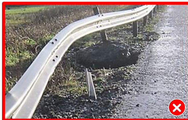
Figure 3.29 - Example of domed concrete foundation which has rotated in the ground, preventing plastic hinge from forming
