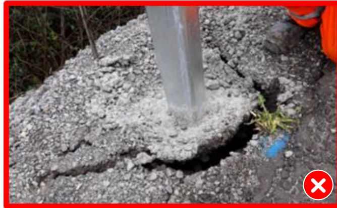
Figure 3.30 - Example of concrete foundation breaking away from edge of embankment due to lack of ground support behind
