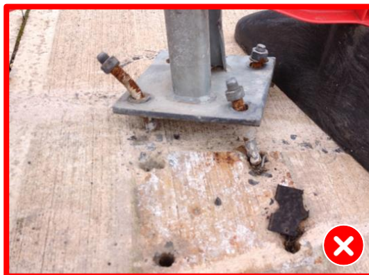
Figure 4.20 - Inappropriate fixing resulted in surface mounted post baseplate pulling away during impact
