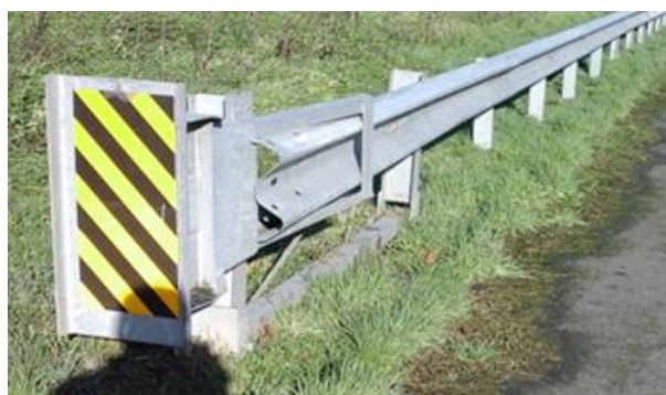
Figure 4.4 - High priority defect: end of beam not tucked into terminal head, poses risk of sparring
