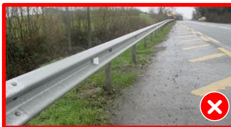
Figure 2.12 - Incorrect reflector colour on nearside verge: should be red facing approaching traffic
