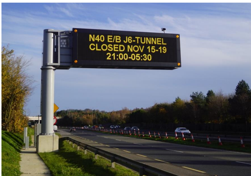
Photograph 4.1 Example of a Strategic VMS (on a Cantilever Gantry)
