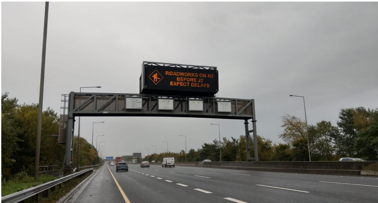
Figure 3.3 Portal gantry mounted VMS
