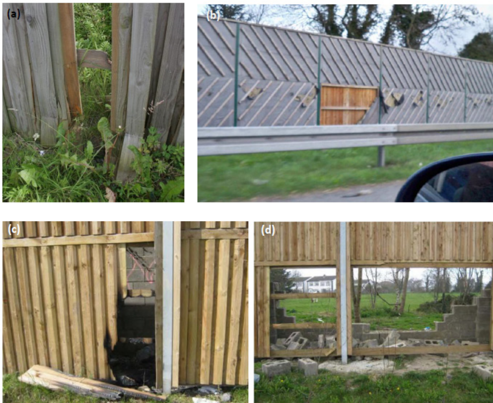
Figure B.23 - Examples of damage to timber noise barriers due to vandalism
