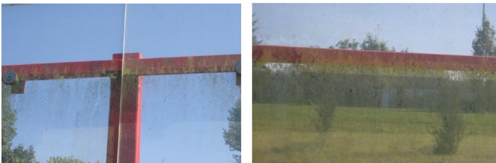
Figure B.19 - Sections of sullied transparent noise barrier
