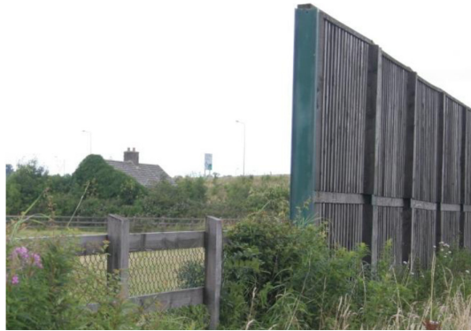
Figure B.5 - Noise Barrier installations where line of sight is blocked but barrier is not long enough to prevent diffraction around sides
